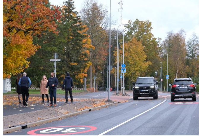
Reconstruction of Sadama Street in Kärkla (contractor: Tariston AS, photo: Eike Meresmaa)
