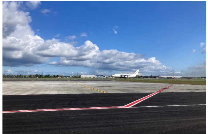
Platform area for Class E aircraft at Tallinn Airport (contractor: Nordecon AS, photo: Koit Kuus)
